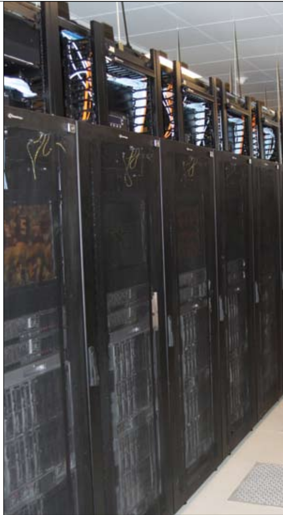
Morgan Kurk of Enterprise Intelligent Buildings, CommScope Inc., believes that data centres at stadiums can also be shared with other companies.
